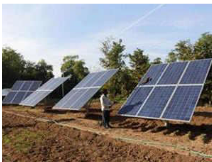
Figure-2 (Solar Panels)
